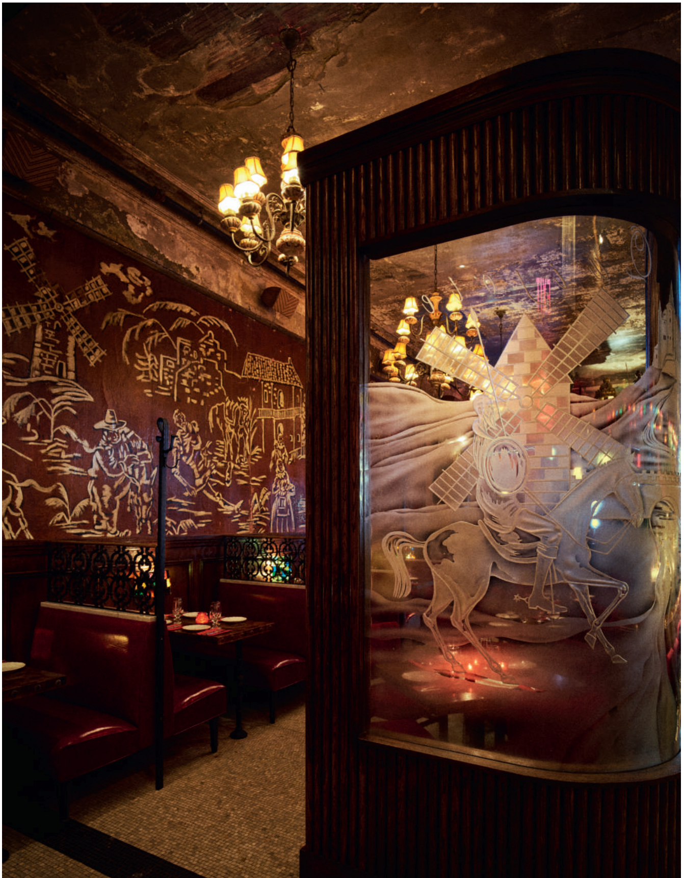
The Don Quixote murals and etched glass depict scenes from Cervantes' epic novel. The banquettes are new, though designed to look as if they are original. A gash in the ceiling, exposing the steel and terracotta beneath the plaster, shows just what a 'light touch' the owners exercised
